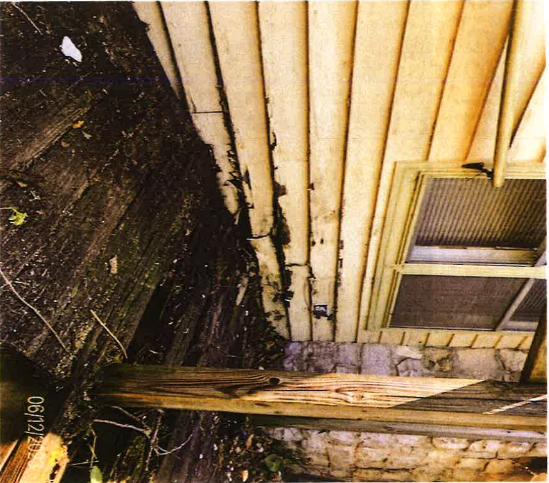
Rear porch decay
